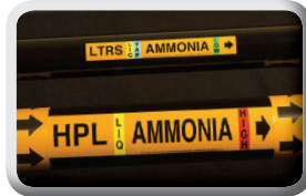
AMMONIA REFRIGERATION MARKERS
