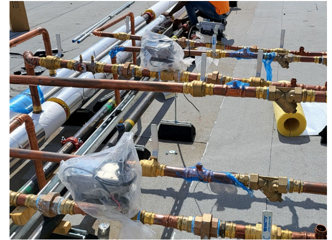
University – Hot Water, Chilled Water, Domestic Water System
